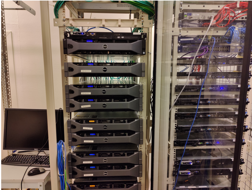
Figure 21: Our server rack at KTH where we run CSLE.
